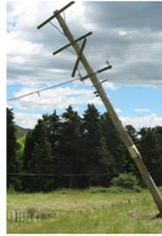
Photo 3: Pole 113116 at failure.
