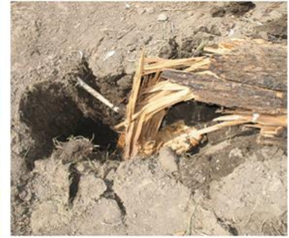
Photo 4: Fracture at ground level at base of Pole 113116.
