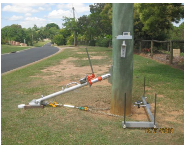
Photo 1: General view of MSPT
