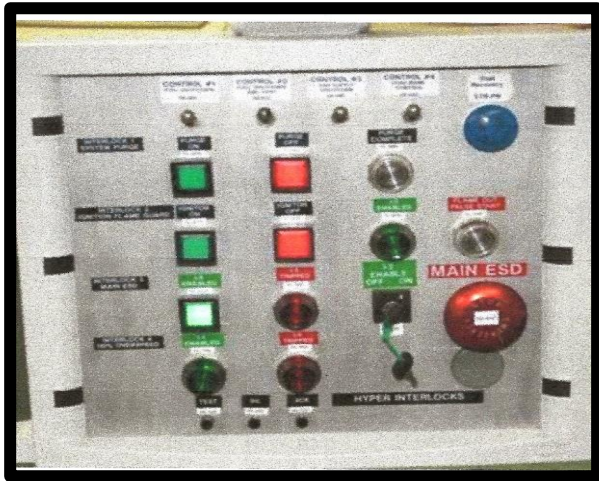
Figure 2 - The Control Panel
