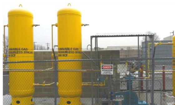
Figure 4: Syngas storage (800 psig) and compressor
