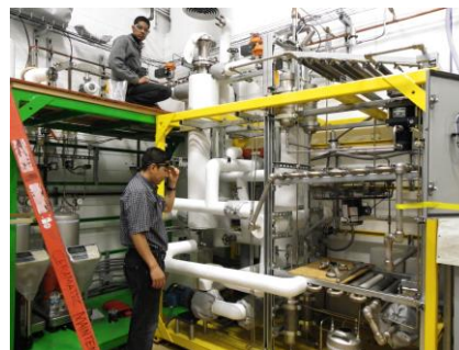
Figure 5: FT reactor system (yellow skid)
