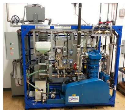
Figure 3: Two-stage compression with cooling
