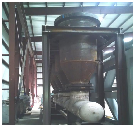
Figure 5: 1 MMSCFD reformers for NH 3 plant
