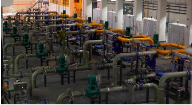
Figure 6: Inside the data center cooling plant rows of pumps flank their associated heat exchanger.
