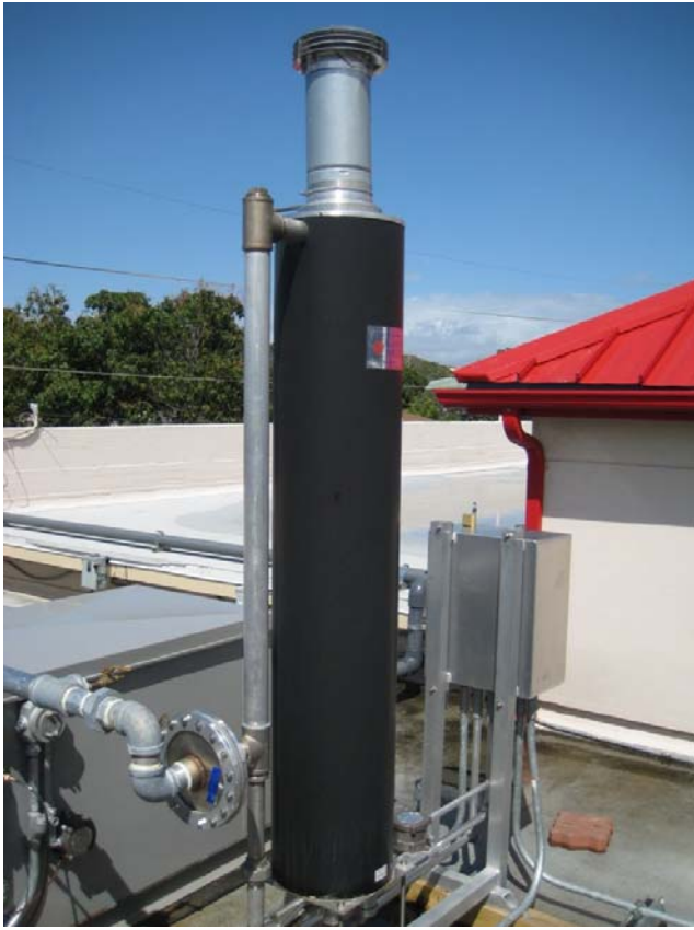
Figure 2: Electric Catalytic Oxidizer Installed On The Roof
