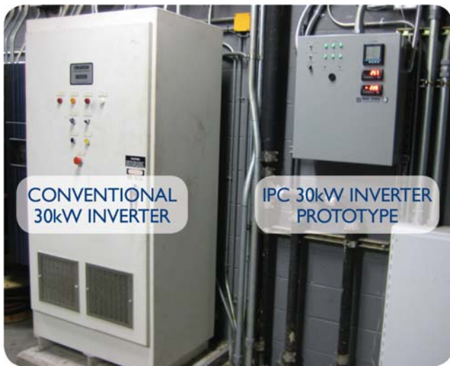
Figure 2. PV Inverter Pilot Installation
