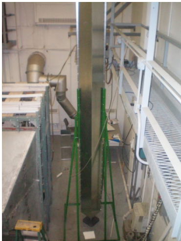
Figure 6. ESP test chamber 3
