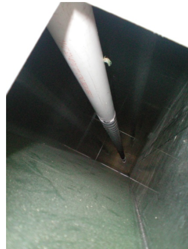
Figure 7. ESP test chamber 3 (inside view)
