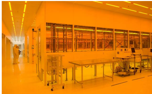
Clean Room – LISE Building Harvard University, Cambridge, MA
