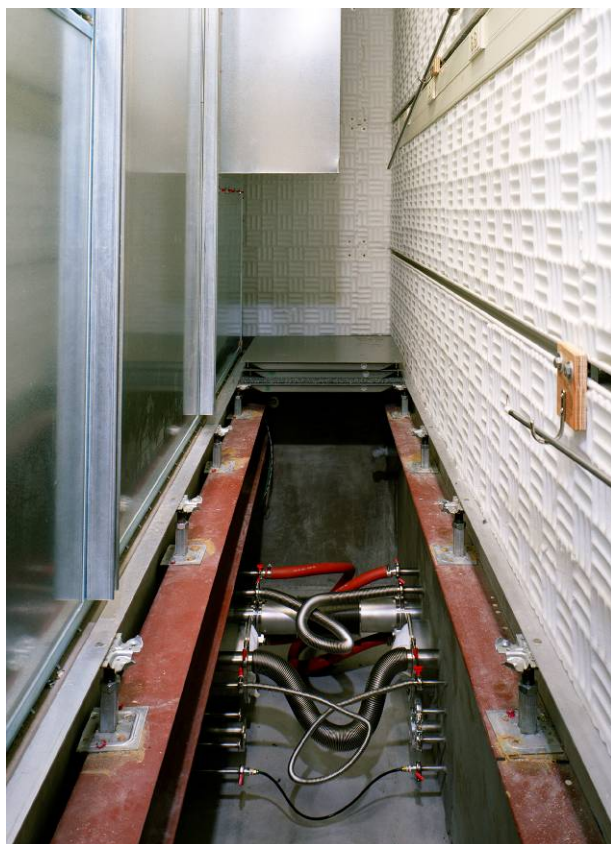
Vibrationally isolated piping and conduit to experiment.
