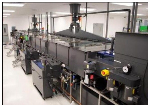
Figure 4. ATMI automated PWB recycling pilot line
