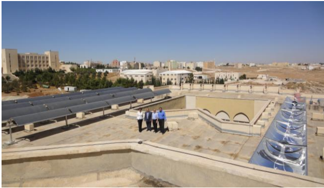
Figure 8: Mu'tah University, Karak Jordan. MicroCSP installation for tri-generation project: electricity, air conditioning and domestic hot water. October 2011
