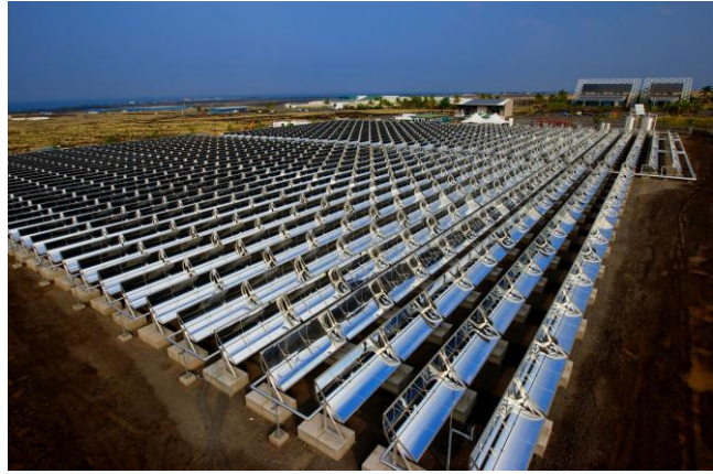
Figure 4: Holaniku, 2 Megawatt Thermal MicroCSP Demonstration Plant in Kona, Hawaii
