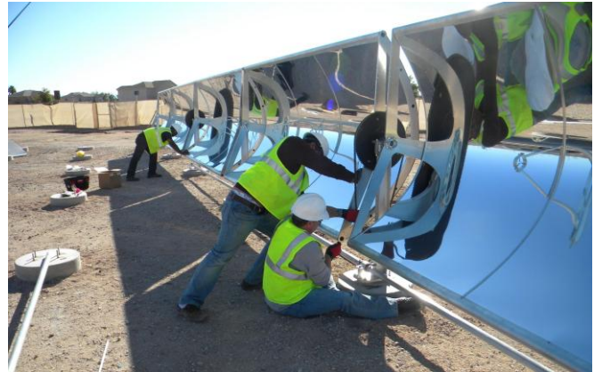
Figure 1: Local labor installing MicroCSP collectors at Davis-Monthan Air Force Base in Arizona.
