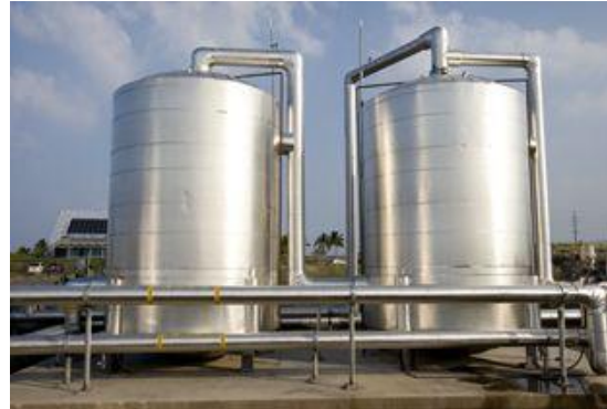
Figure 8. Thermal storage at Holaniku, Kona, HI
