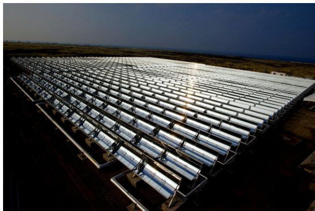
Figure 2: Holaniku 2-megawatt thermal solar field
