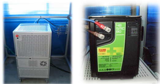
Figure 2 SOFC system (SOFCpower/Dantherm Power) and Fiamm SoNick 48TL80-NV during tests at CNR-ITAE
