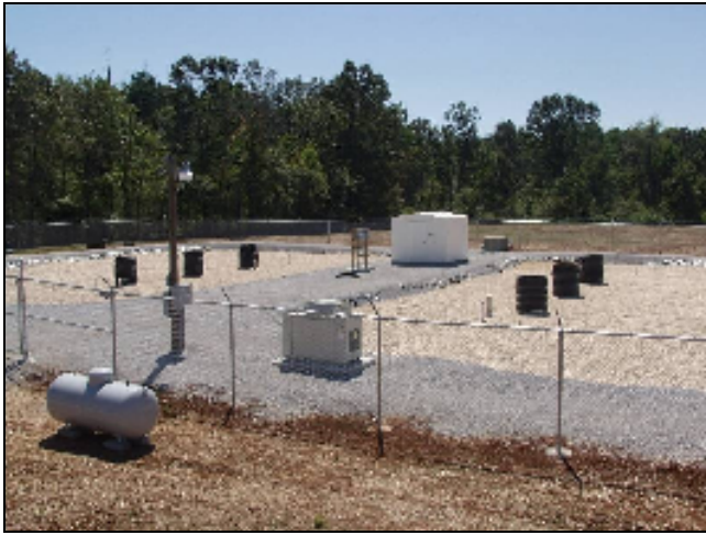
Figure 3. Commercial 40,000 gal/day sanitary wastewater ReCip® system installed at the Barton Riverfront Industrial Park, Barton, Alabama. The black upright cylinders are pump chambers to house axial flow pumps. This system is operated as a gravel-only system with no plants.
