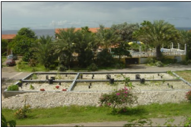
Figure 4. Four-cell ReCip® "Water Garden" installed at Sunset Beach Diving Resort on the desert island Curacao. The system treats up to 5000 gallons of clarified wastewater each day. The clear and odor free wastewater is used for irrigating landscape plants, while excess water is sold to water vendors who resell the treated wastewater for irrigation
