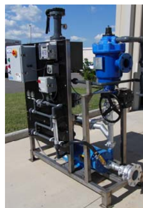
Figure 2. A Standard CHC Unit with a Separator System and Controls
