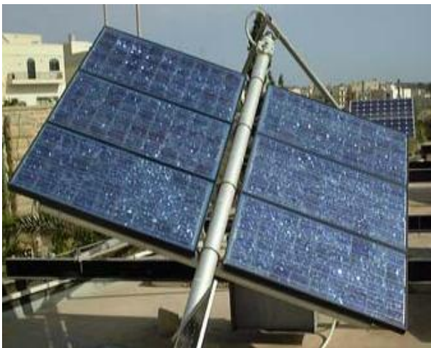
Figure 3: General view of PV generator.
